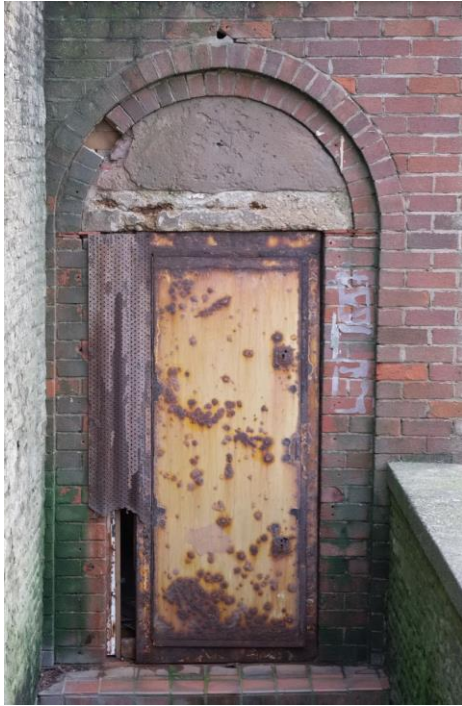
Badly rusting security doors to disused toilets under Promenade lift entrance
