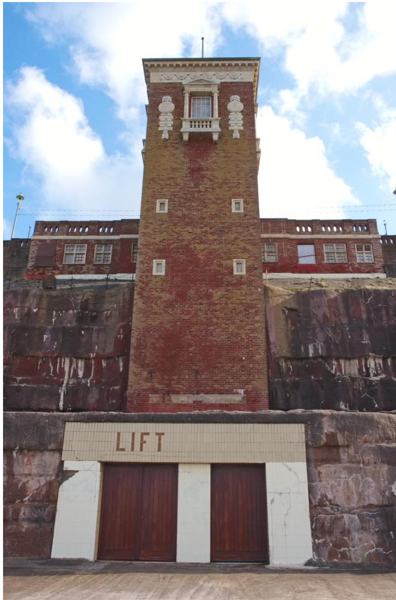
Entrance to non-functioning lift from Lower Walk
