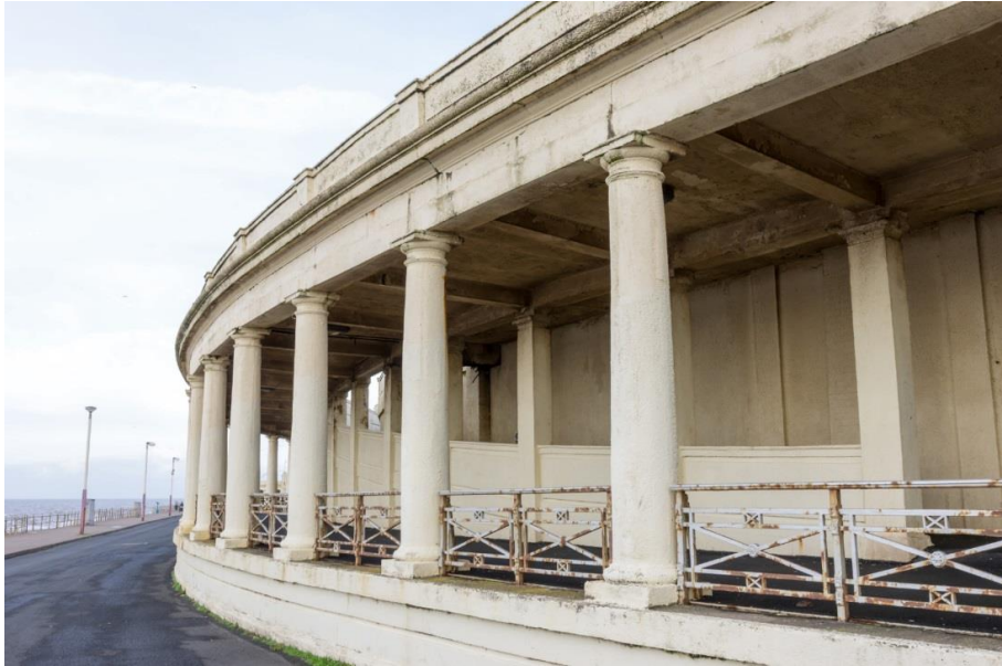
Railings in need of repainting
