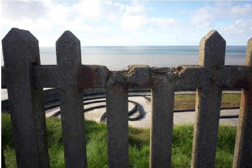
Broken and corroding concrete fencing
